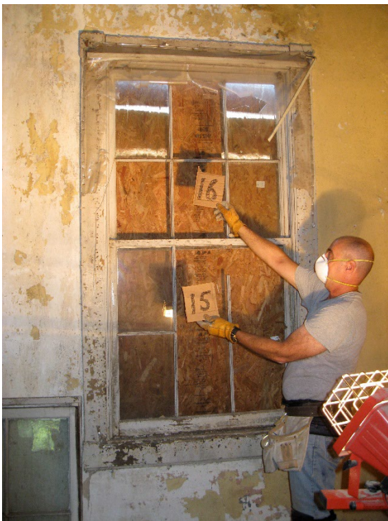
Window "A" from interior, north elevation, showing damaged and missing muntins in both sash which will be recreated.
